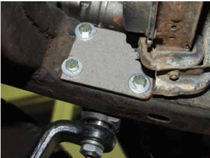
This photo shows a simple frame repair using steel plate. (not provided)
